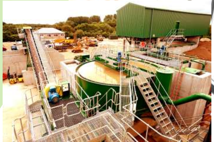
CDW separation and recycling facility
